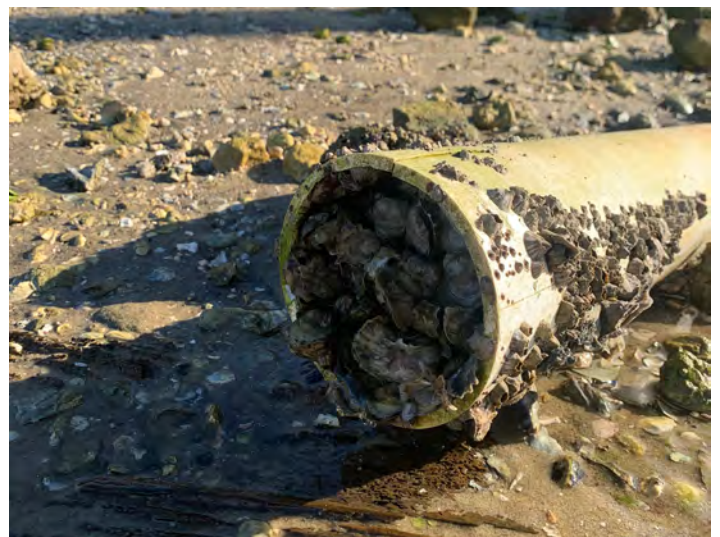
Figure 2: Drainage pipe. Photo credit: Thomas Ruppert
